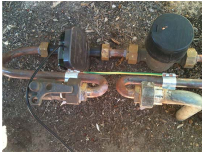
Figure 2.3: Installation of Aquiba A200 meter (left with optical sensor for manual download attached) in series with existing SA Water meter (right)
